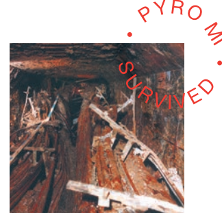
Pyro MI survived in this power station fire
