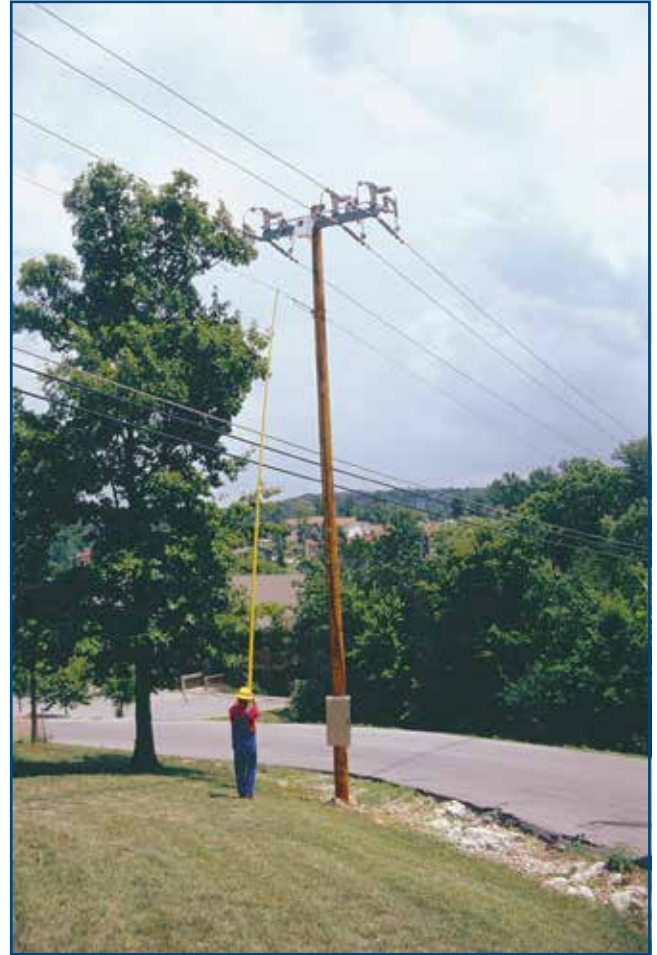
Clean and uncluttered appearance . . . sensors, control power source, and a three-phase disconnect are built-in.
