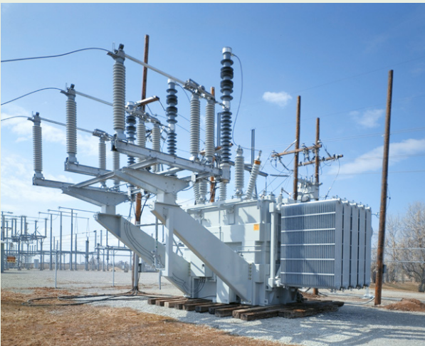
FIGURE 6. A 138-kV Model SE Trans-Rupter II Transformer Protector mounted to transformer at a temporary installation on railroad ties.
