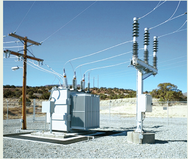
FIGURE 8. A 69-kV Model SE Trans- Rupter II Transformer Protector on an S&C Mounting Pedestal.
