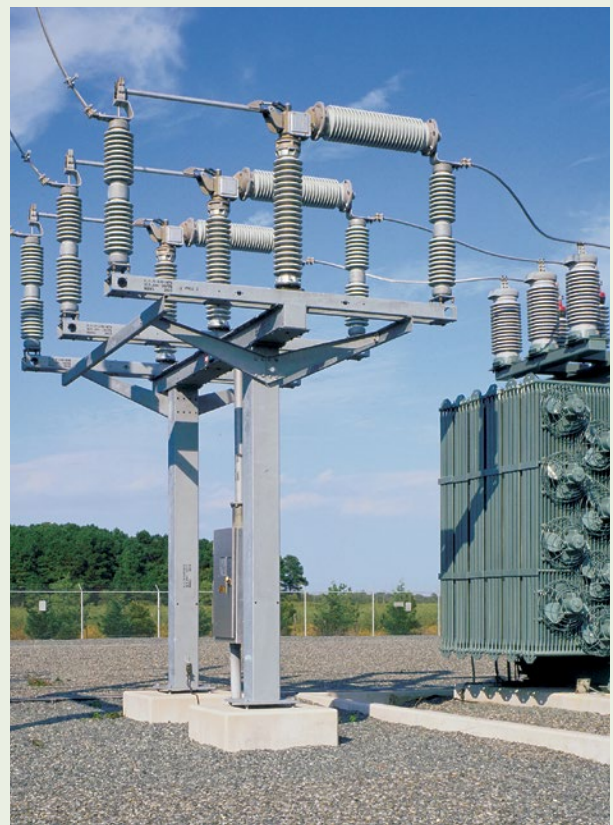
FIGURE 1. A 138-kV Series 2000 Circuit-Switcher Model 2010 with horizontal interrupters and a vertical-break disconnect.
