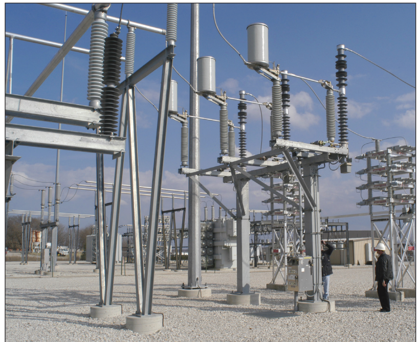
138-kV Mark VI Circuit-Switcher on S&C Mounting Pedestals.
