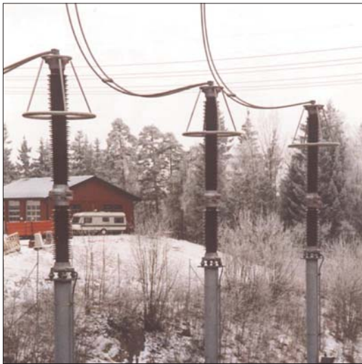
220 kV Surge Arresters - Norway
