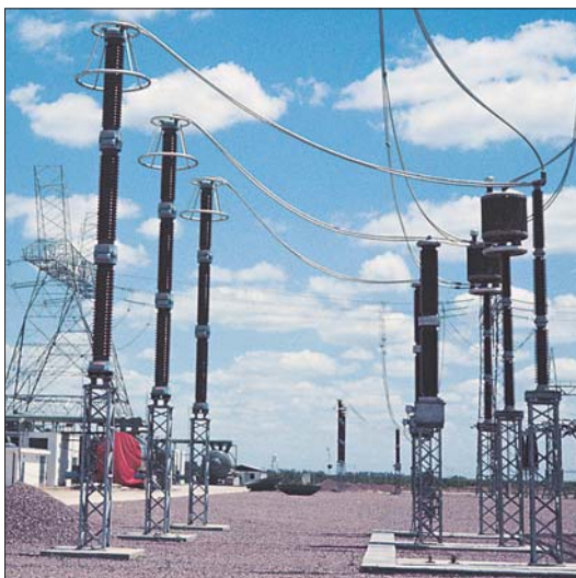
300kV Surge Arresters - Kuwait
