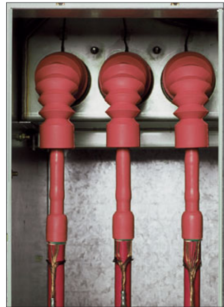
IXSU-F terminations installed with Raychem elastomeric bushing boot (RCAB)
