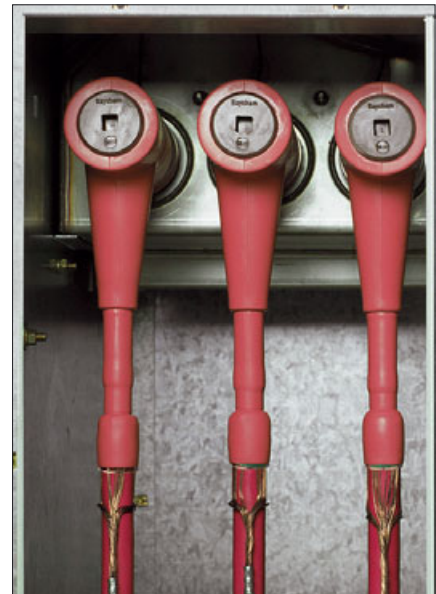
IXSU-F terminations installed with Raychem insulated connection system (RICS)
