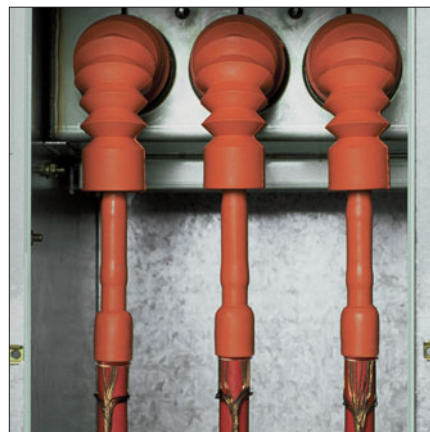
TFTI installed with Raychem bushing boot (RCAB)
