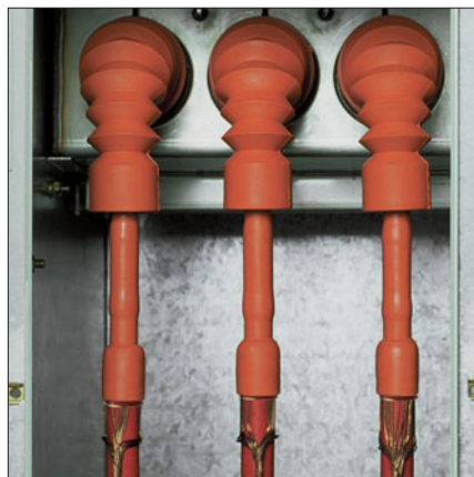
TFTI installed with Raychem bushing boot (RCAB)
